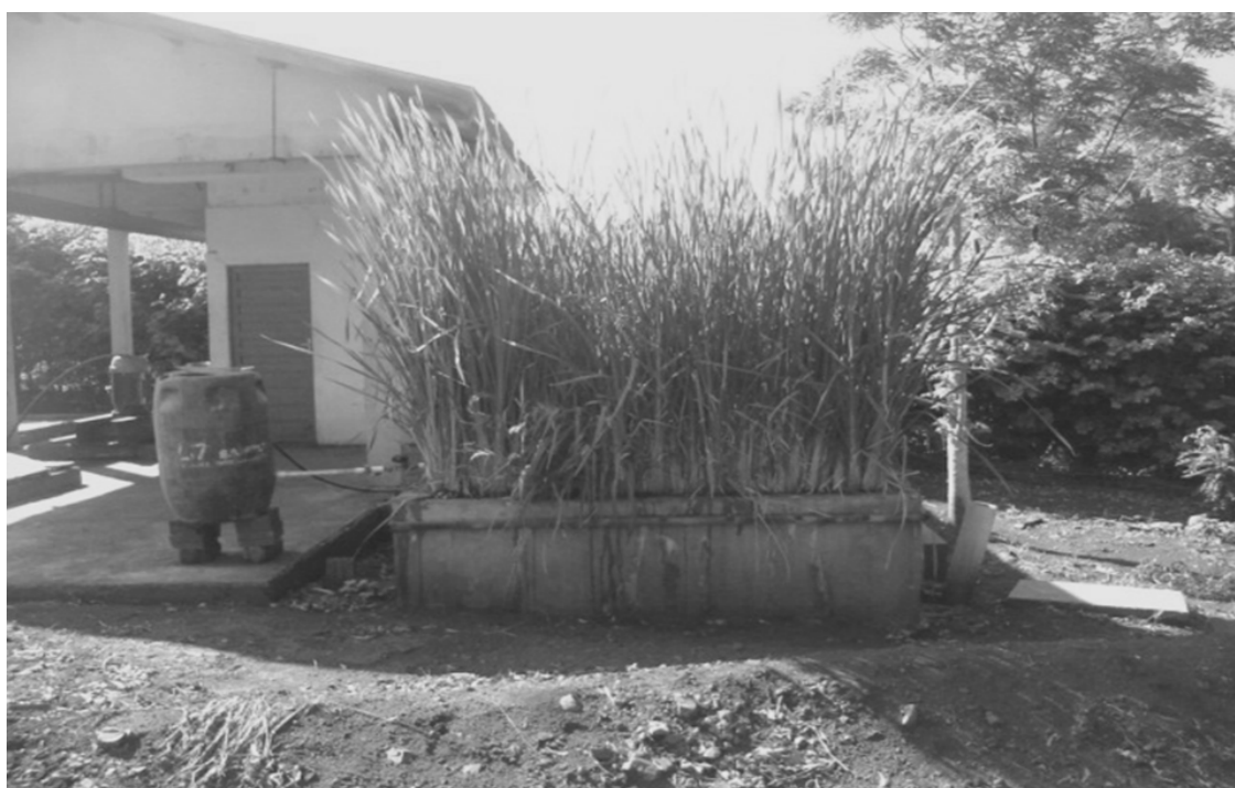
Figure 1. Constructed wetland system of horizontal flow installed in stabilization pond (sewage treatment station of Bandeirantes-PR, Brazil). On the left, there is the reservoir connected to the hydraulic loading rate (HLR) control.
