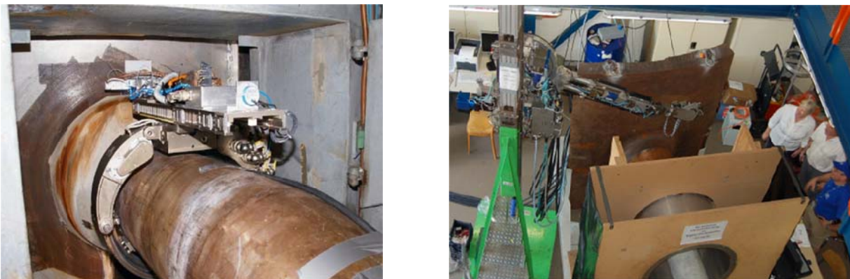
Figure 4. Reactor pressure vessel nozzle inspections on-site (left) compared to practical demonstrations in the qualification process (right).
